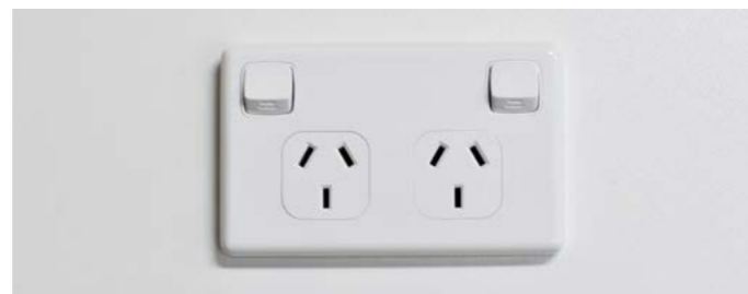
Shaving Cabinet Power Point
